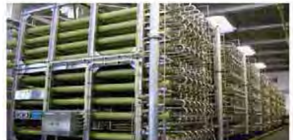
Photo: Interior of a seawater desalination facility (Okinawa Enterprise Bureau Chatan Water Purification Plant)
