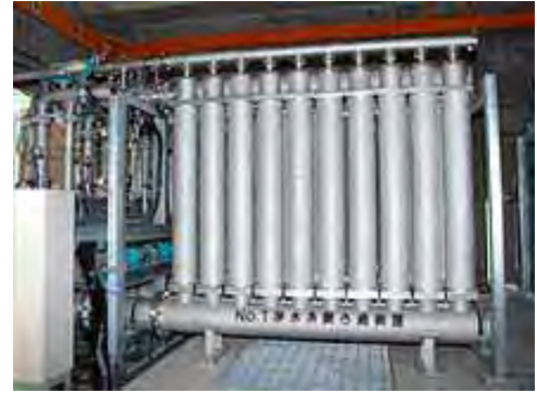
Photo: Membrane filtration system (From METAWATER Co., Ltd. HP)
