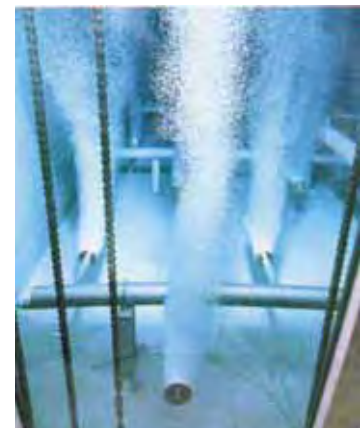
Photo: Ozonation plant (Tokyo Kanamachi Purification Plant)
