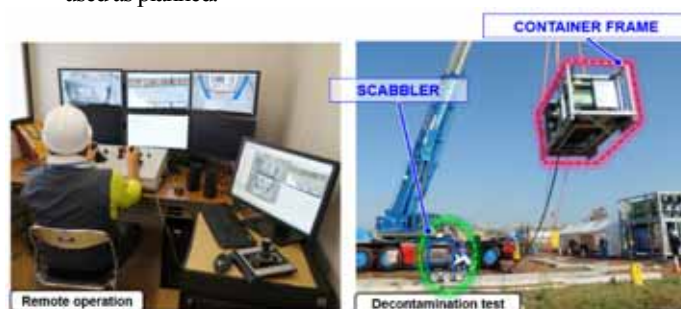
Decontamination equipment: The system is operated from a remote operation room using a camera equipped on the scabbler.
