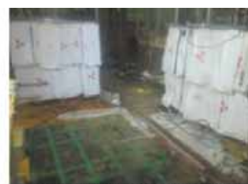
L-shaped temporary shielding
