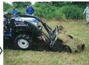
A front loader was used, the soil was scooped up and removed.
