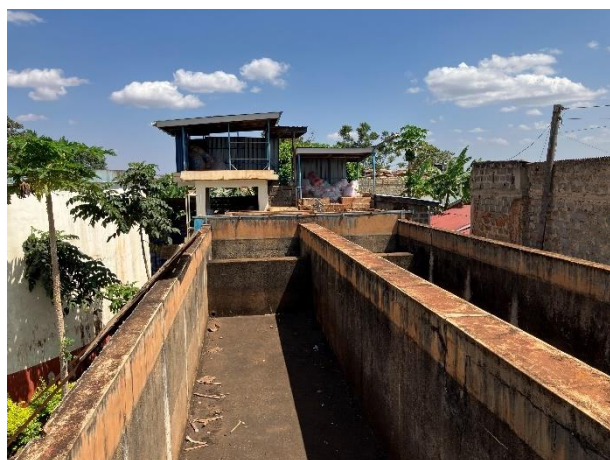
Photo 2-22 Kiharu WTP (Horizontal-flow Sedimentation Basin)
