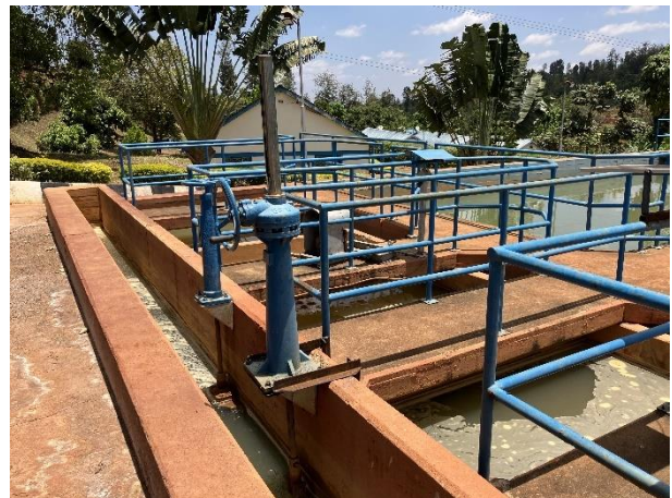
Photo 2-15 Mechanical Slow Mixing
