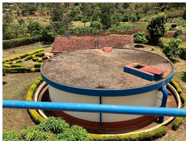
Photo 2-21 Clear Water Reservoir (370 m 3 )
