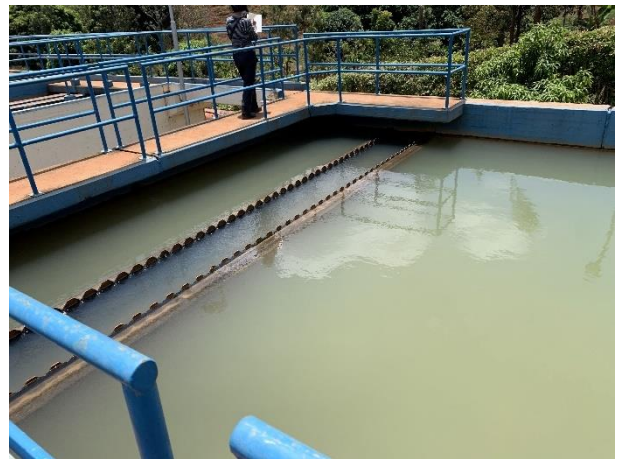
Photo 2-17 Horizontal-flow Sedimentation Basin (Outlet Part)
