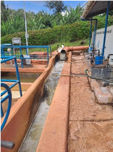
Photo 2-14 Receiving Well and Rapid Mixing by Hydraulic Jump
