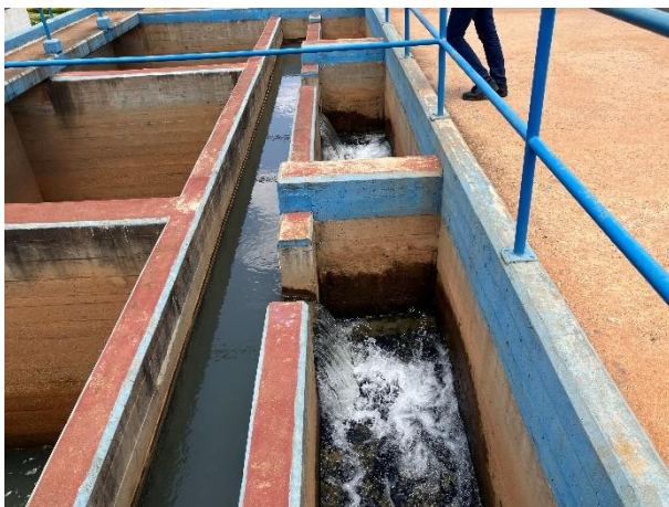
Photo 2-18 Rapid Sand Filter (Inlet Part)
