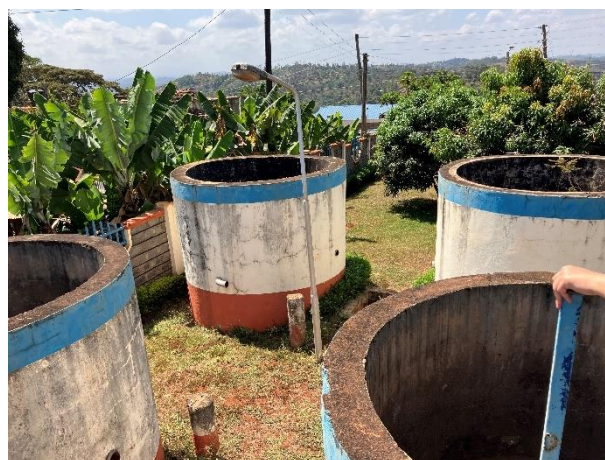
Photo 2-23 Kiharu WTP (Rapid Sand Filter)
