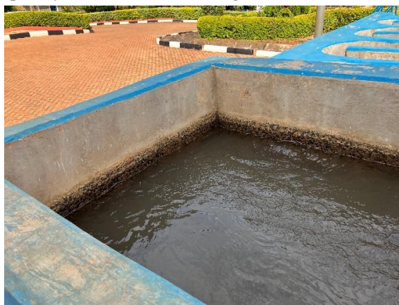
The water level at the receiving well during the capacity verification
