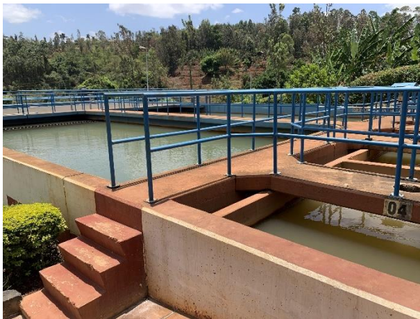
Photo 2-16 Horizontal-flow Sedimentation Basin
