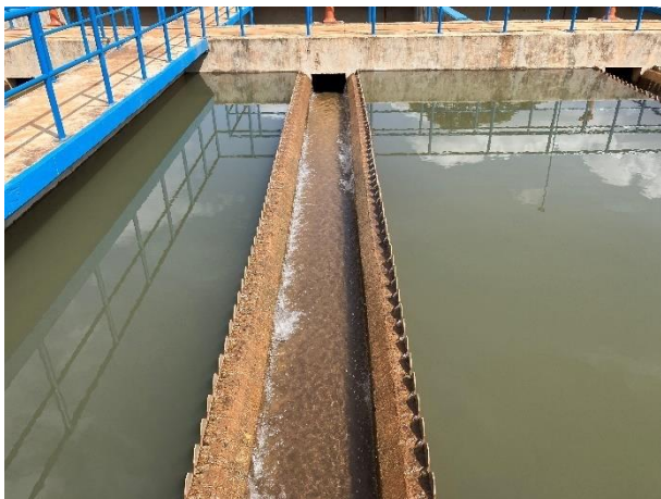
Photo 2-8 Horizontal-Flow Sedimentation Basin (Outlet Trough)
