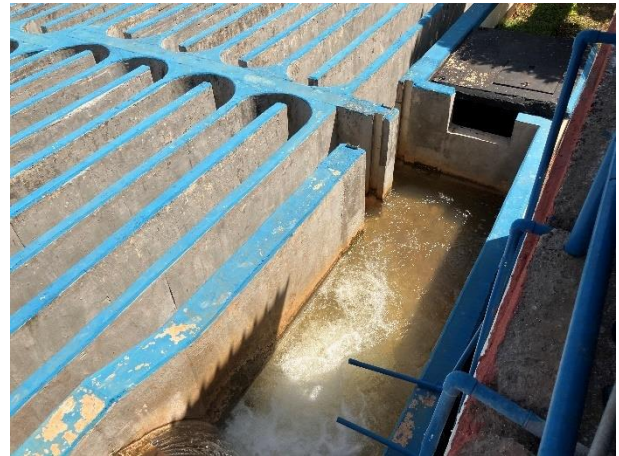
Photo 2-7 Horizontal-Flow Flocculator with Baffled Walls (Inlet Part)
