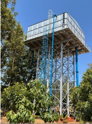
Photo 9: Elevated Water Tank (Kiawambeu WTP)
