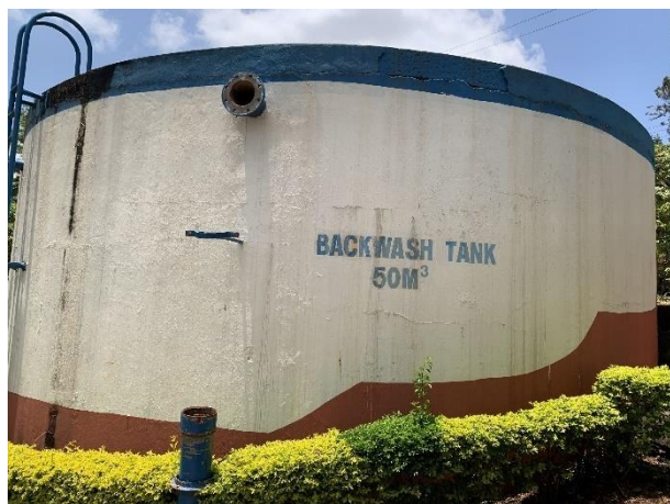
Photo 2-20 Backwash Tank (50 m 3 )
