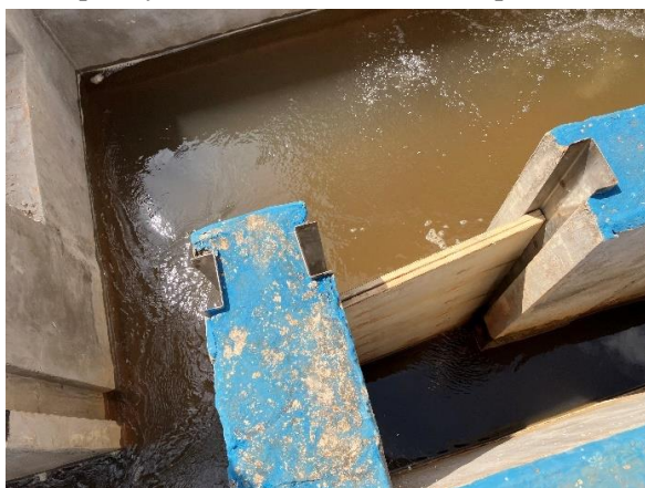
The installation status of the stop-log at the inlet of the flocculator
