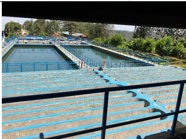
Photo 6: Flocculator and Clarifier (Kiawambeu WTP)
