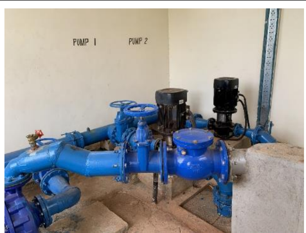
Photo 10: Pump Room (Kiawambeu WTP)
