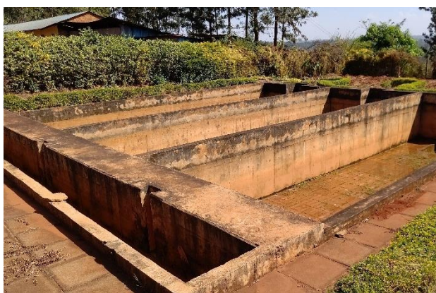
Photo 2-12 Sludge Drying Beds
