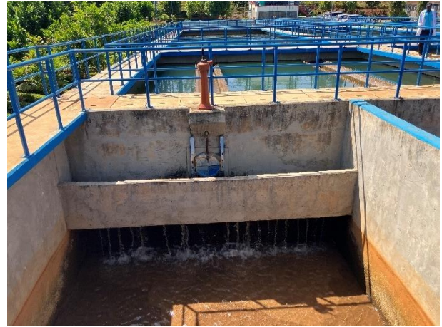
Photo 2-9 Rapid Sand Filter (Inlet Part)
