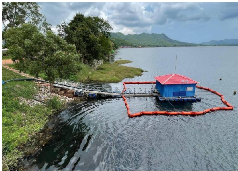
Figure 4: Water Intake at the Mech Water Treatment Plant in Kampot Province (provided by Kobelco Eco-Solutions Co., Ltd.)
