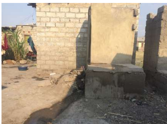
On-site sanitation facilities in the Garden Park area
