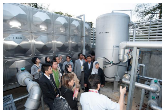
Water cistern tanks
