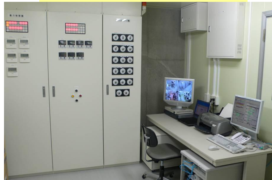
3. Monitoring & Management Room
